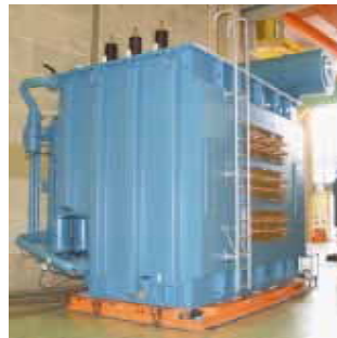
160 MVA steel EAF Transformer. Internal closure.
