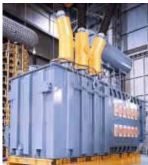
79 MVA Rectifier Transformer. Common tank.
