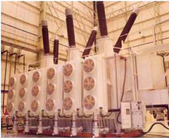
450 MVA auto-connected system intertie transformer
